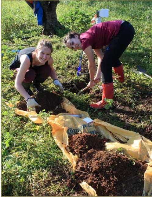
Figure 2: Installing moisture sensors at a golf course within the Costa Nabvarino resort.
