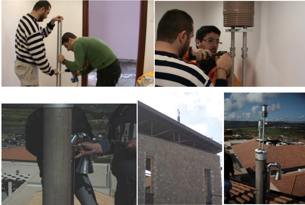
Figure 1. Installation works at the Library Tower and the final inlet setup on top of the roof.
